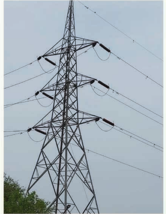
Bird diverters installed on powerlines falling in GIB sensitive habitats Courtesy: Spring
